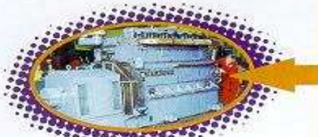
Figure 11: 250 kW Dual fuel diesel engine modified by Ormrod Diesels, UK, to run on bio-oil
